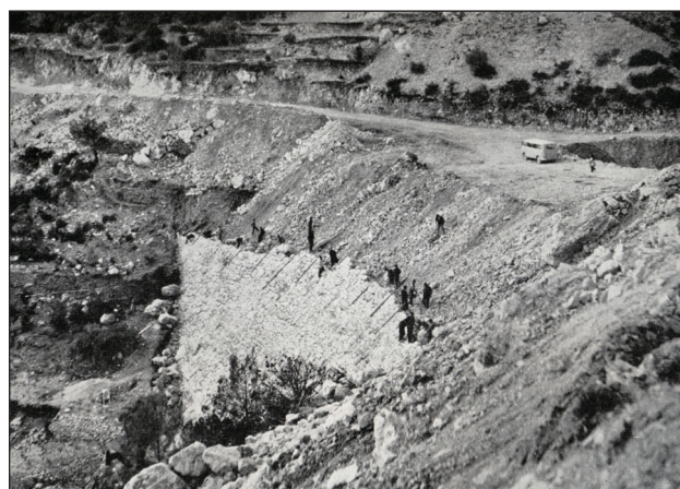
Figure 6: The cladding of slopes in hand-bonded broken local stone. From Kečkemet (1965: 48); photographer unknown.
