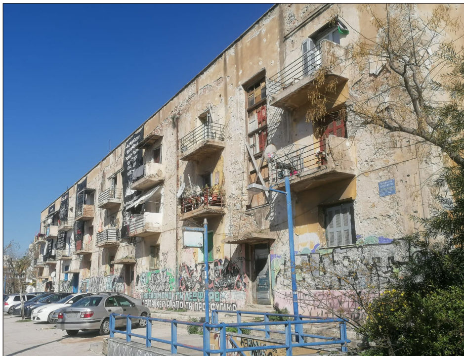
Figure 22: The Prosfygika building complex on Alexandras Street today. Photo by Stelios Gidis, 2024.
