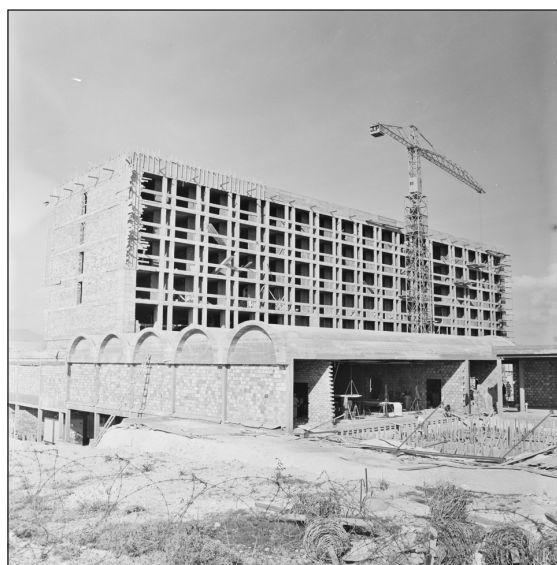
Figure 4: The Hilton Hotel under construction, circa 1968. Courtesy of Press and Information Office, Nicosia.
