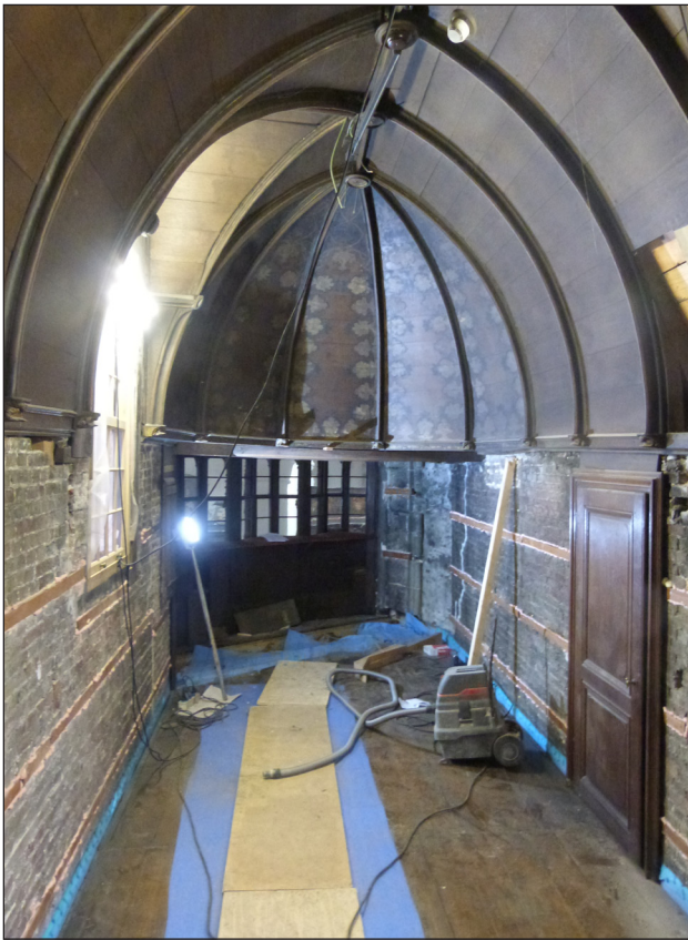
Figure 10: The gallery of Louis of Gruuthuse in his residence at Bruges. Photo taken by Sanne Maekelberg during restoration.
