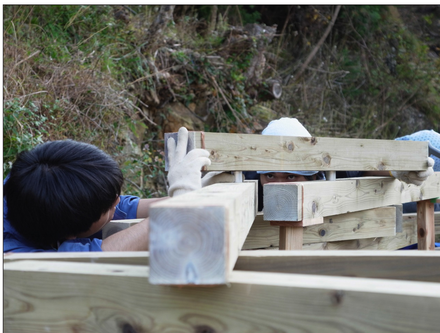
Figure 12: Kozumihama Ojizō-sama Project, Ishinomaki, 2013. Construction by Hosei University students. Watanabe+Shimohigoshi Independent Studio. Photo by Hiroyuki Hirai.
