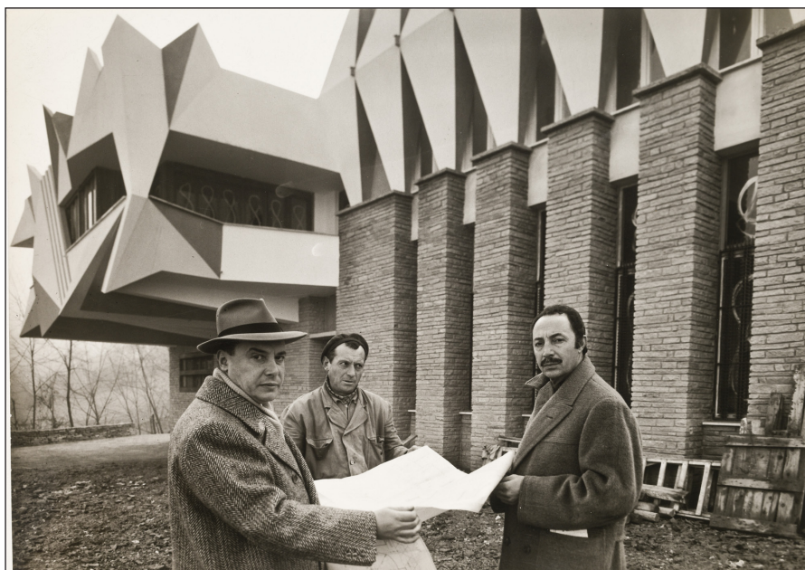
Figure 5: Enzo Venturelli (left) and Umberto Mastroianni (right) at the construction site of Casa Mastroianni, circa 1955. AEV b.12 © Archivio di Stato di Torino.
