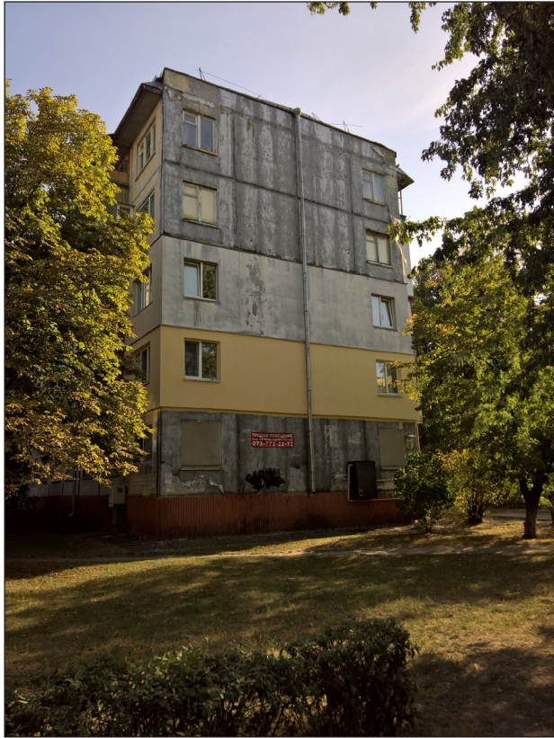
Figure 11: Prefabricated panel buildings with individual, user-installed insulation on the façades in Darnytsia (Pivnichno-Brovarskiy massyv) and Voskresenka neighborhoods in Kyiv, Ukraine, current condition. Photos by Kateryna Malaia.
