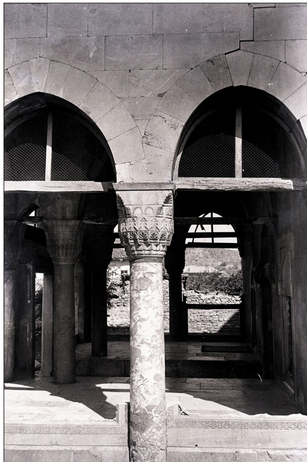
Figure 12: Lateral column of the portico. Photograph taken in 1938 or earlier. ASÜA, SALT. https://archives.saltresearch.org/handle/123456789/205660 .
