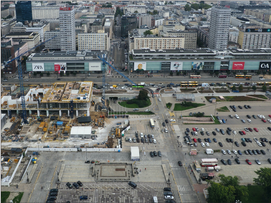
Figure 10: Museum of Modern Art Warsaw and TR Warszawa Theater on Plac Defilad under construction, view from the Palace of Culture and Science. Architect: Thomas Phifer and Partners, New York. Client: Museum of Modern Art in Warsaw. Photo by Alicja Willam, 2021 © CC BY 2.0.
